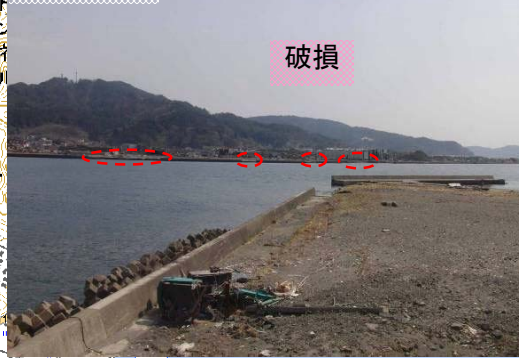
⑧堤防破損
