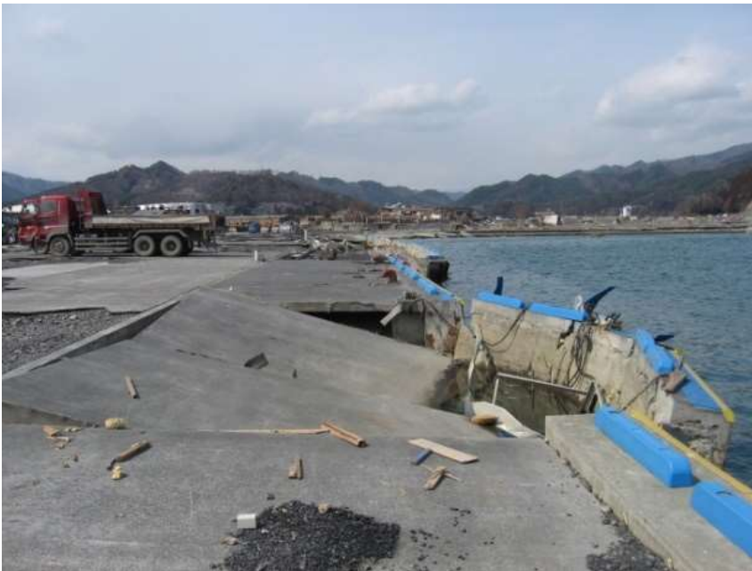
Damage to the Quay (Otsuchi Fishing Port)
