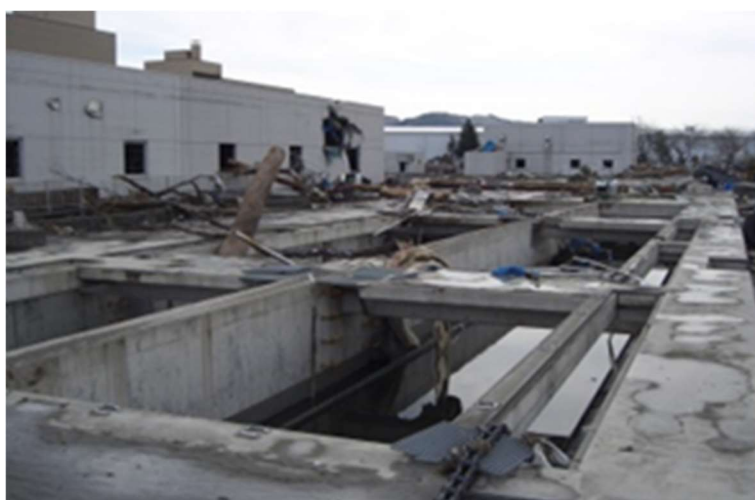
Ofunato Septic Center
