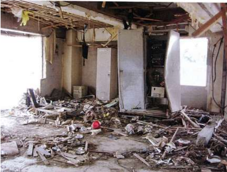
Central Control Room Damage (Rikuzentakata City)
