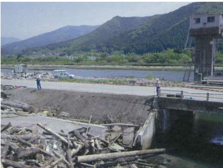
Auxiliary Pipe Damage (Ofunato City)
