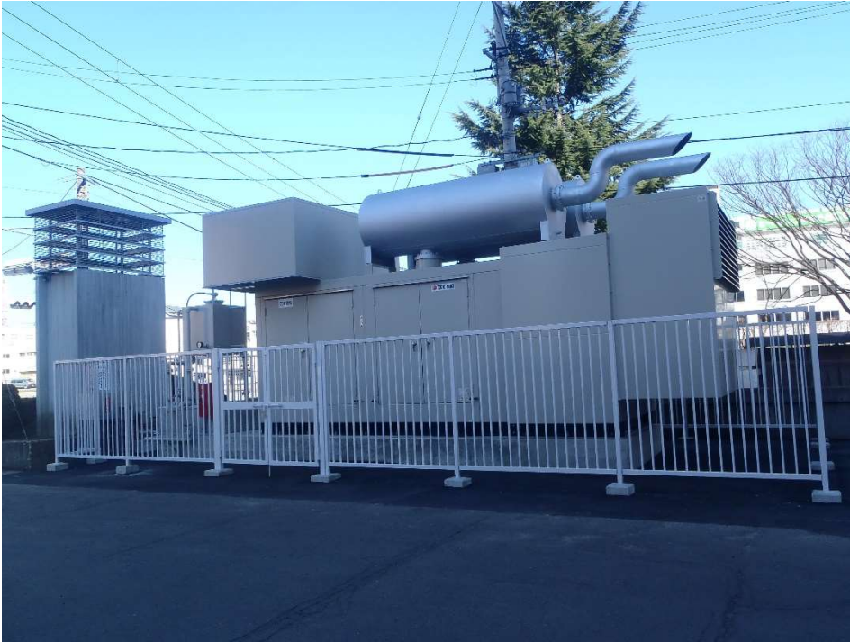
Renewed emergency power generation equipment at the Morioka District Joint Government Office Building (maintenance completed in the 2013 fiscal year)
