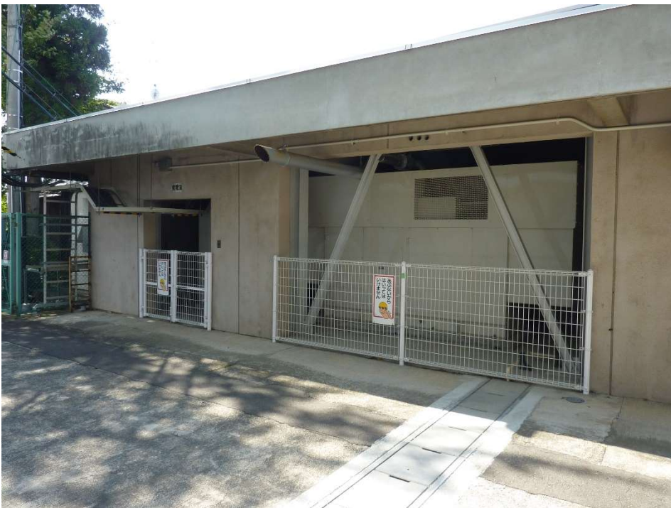
New installation of emergency power generation equipment at the Oshu District Joint Government Building (maintenance completed in the 2012 fiscal year)
