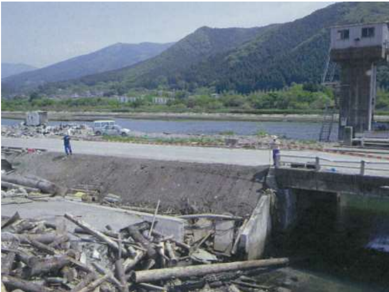
Auxiliary Pipe Damage (Ofunato City)
