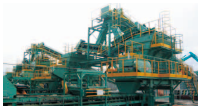
Tsunami sludge treatment facility in Rikuzentakata
