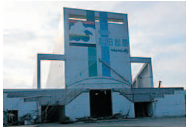
Disaster Site (Takata Matsubara Road Station, which took extensive damage in the tsunami)
