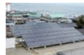
Solar power facility installed on the roof of the Hirono Town Hall
