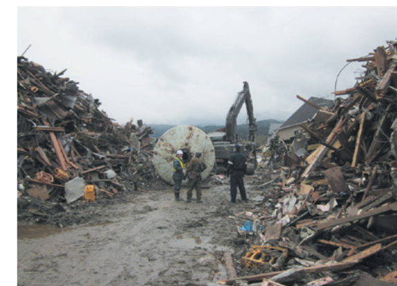
The road clearance work in Rikuzentakata City (Source: Rikuzentakata City, Iwate Prefecture)
